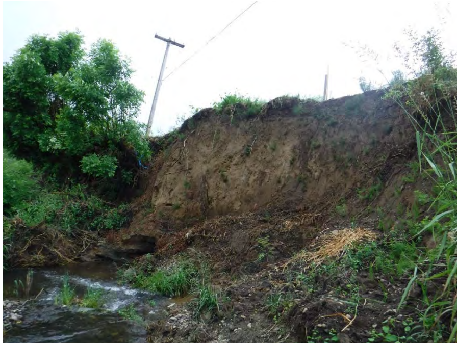
Photo 2. Eroding bank showing erosion from flow redirected by fallen tree.
