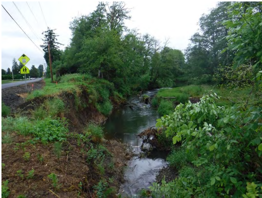
Photo 3. Eroded bank slope, looking upstream from top of bank. Photo taken on 6/8/2017.
