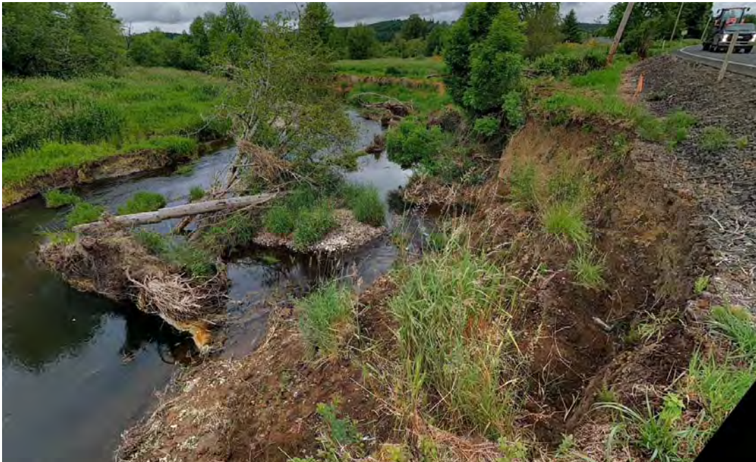
Photo 1. Eroded bank slope, looking downstream from top of bank. Photo taken on 6/8/2017.
