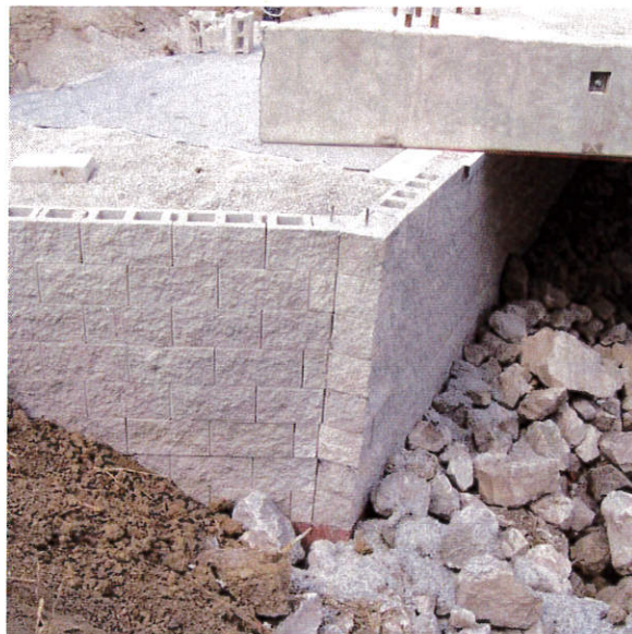
Figure 58. Photo. Vertical seam in wing wall.
