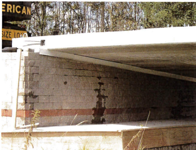
Figure 70. Photo. Aluminum flashing (drip edge) between beams and top of CMU block.
