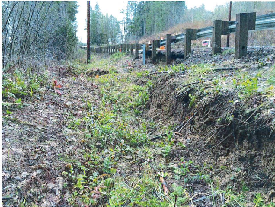
Photo 3. Looking west along scarp from below
