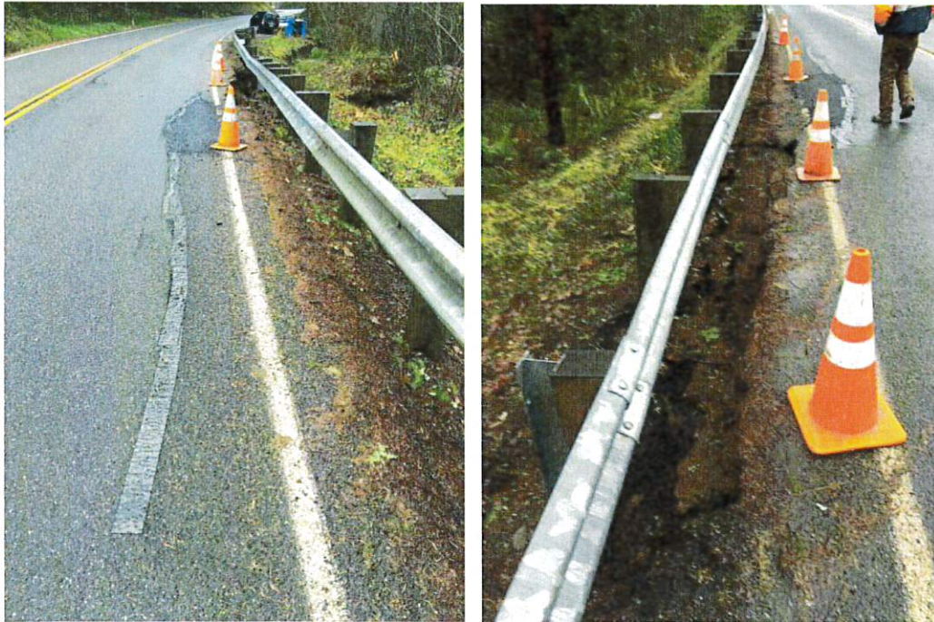
Photo 1. [Left] Looking east at pavement cracks and scarp. [Right] Looking west at scarp
