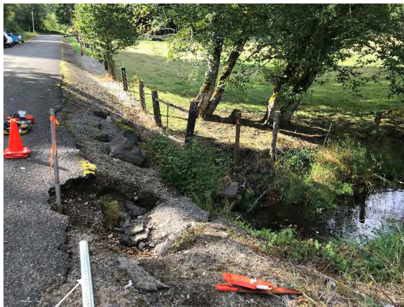
Figure 18 View of the eroding roadway crossing above the culvert outlet (Station 25+50, white arrow indicates flow direction)
