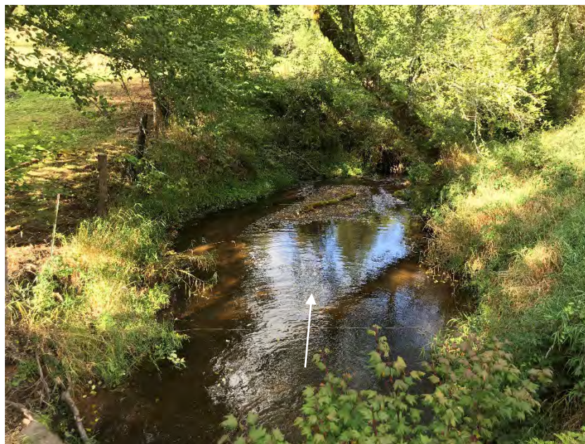
Figure 19: Channel conditions immediately downstream of the culvert outlet as seen from the roadway, with the deep scour pool transitioning into a transverse bar near at the channel bend (Station 25+50, white arrow indicates flow direction)
