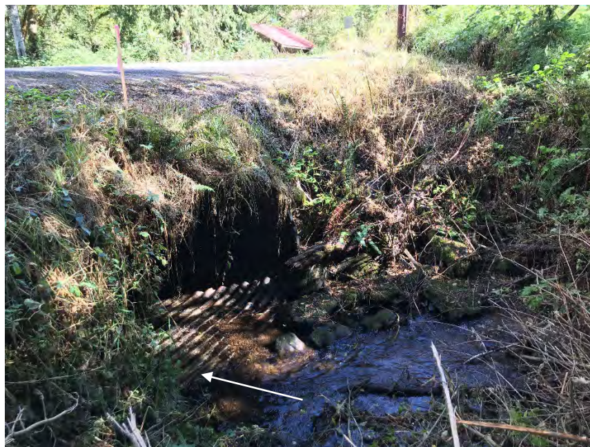
Figure 14: Conditions at the culvert inlet, including eroded roadway fill and a lack of alluvial cover on the culvert bottom (Station 25+00, white arrow indicates flow direction)
