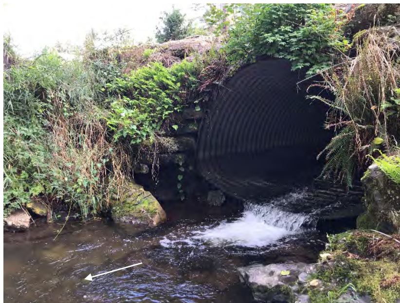
Figure 20 Existing conditions at the culvert outlet, showing a water surface drop and exposed bedrock in the nearby banks and below the culvert itself (Station 26+00, white arrow indicates flow direction)
