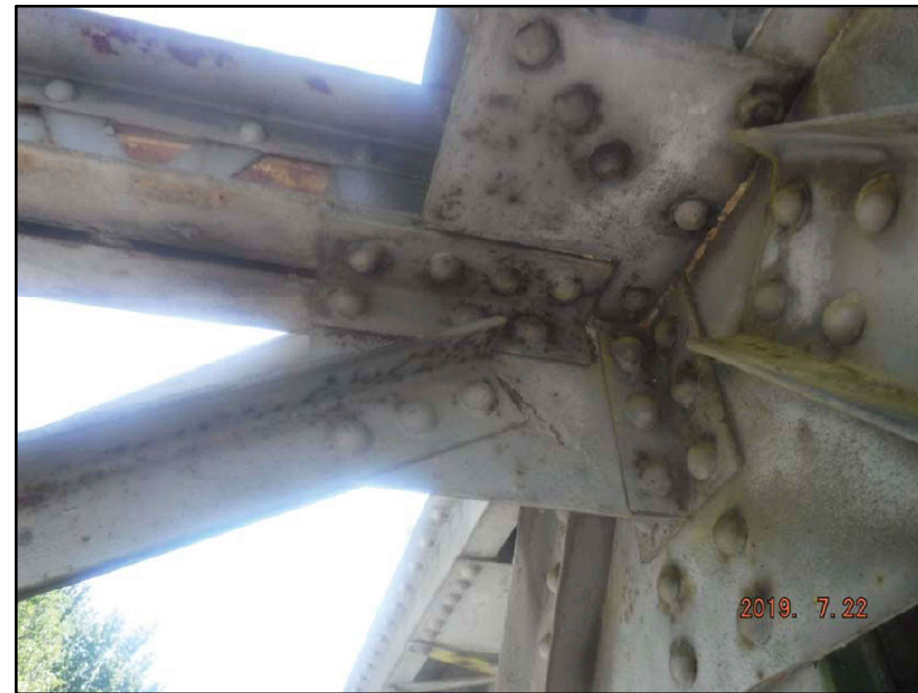
SI-33: U3 SWAY IMPACT DAMAGE POPPED PAINT IN TOP CHORD PLATE CONNECTION
