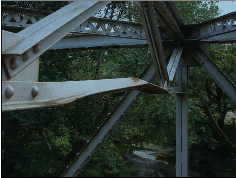
SI-13: IMPACT DAMAGE TO U3-U3
