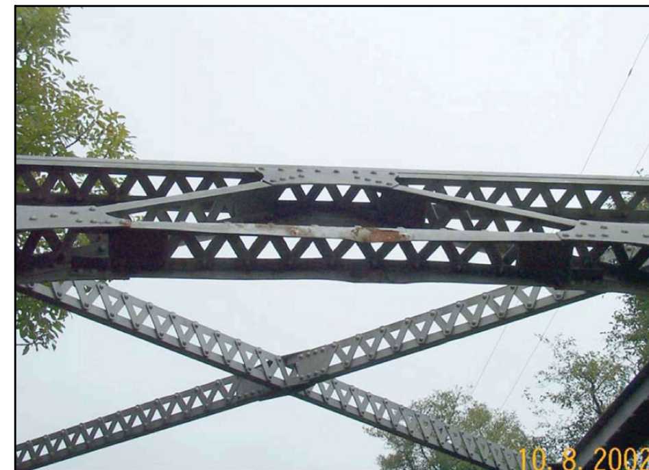
MI-6: IMPACT DAMAGE TO U1 (WEST) PORTAL LOWER CHORD
