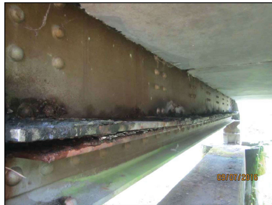
SI-19: ACTIVE CORROSION/PITTING IN FLOOR BEAM WEB
